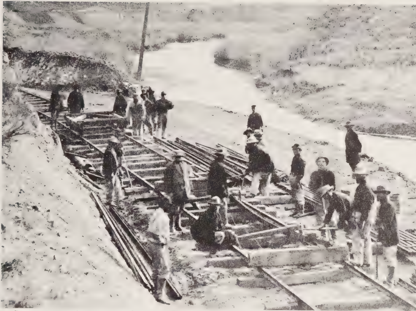
Construction Gang of the Central Pacific Curving the Iron Rails by Hand with the Aid of Heavy Hammers
